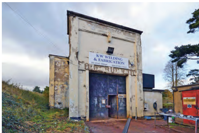
Maintenance Building 58 was one of two buildings on the site used for the inspection of bombs brought from the airfields (called Maintenance and Repair Building on the plan). It was a drive through building, with large double height steel doors at each end, and thus didn't need overhead gantries. A concrete retaining wall at the left of the picture provides a cutting and curved traverse through one of the earth berms. This view shows the large entrance doors at the east end. This building used to have a RAF Police watchtower on its roof
